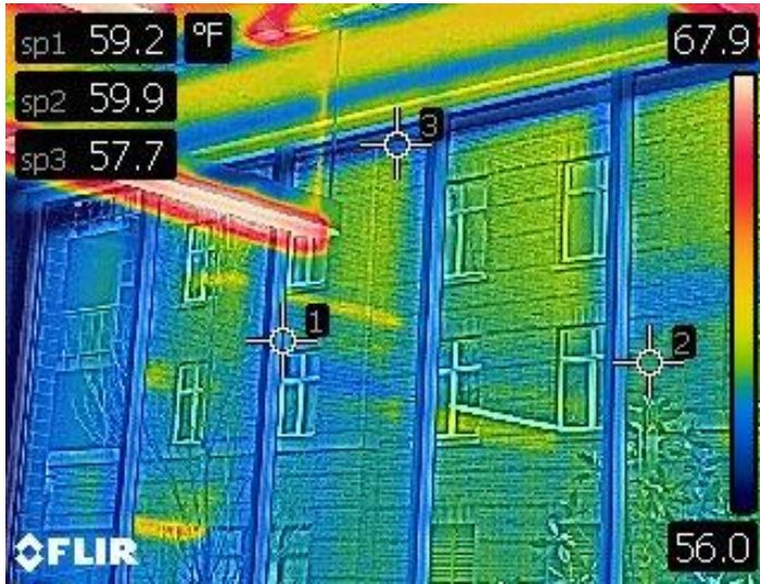
G.L. - Bike Window Type- Curtain Wall FLIR Thermal Image: Data Collection Day #1
